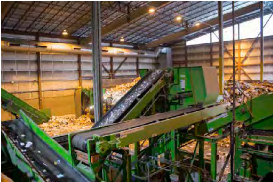
Recology CleanScapes materials recovery facility
