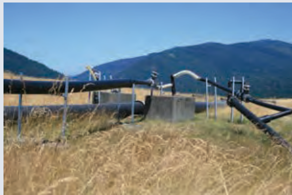
Gas collection pipes at the Cedar Hills landfill
